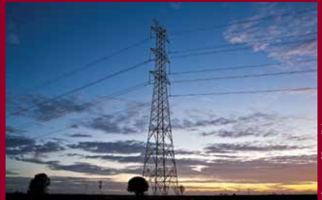
Courtesy of Powerlink
